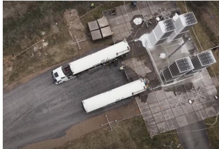
Engineered solutions to meet specific requirements Example 33Mt H 2 over 5 days & peak flow rate : +15 kNm 3 /h
